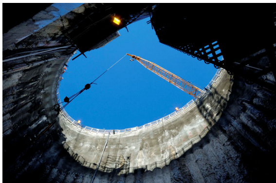
Figure 2: Starting shaft established in the Copenhagen limestone in level minus 35 m for TBM activities.
