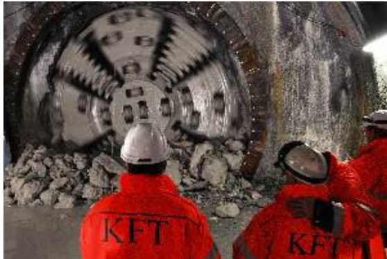
Figure 1: Breakthrough of the 5.1 m Herrenknecht TBM for a new service tunnel for district heating in the city center of Copenhagen.
